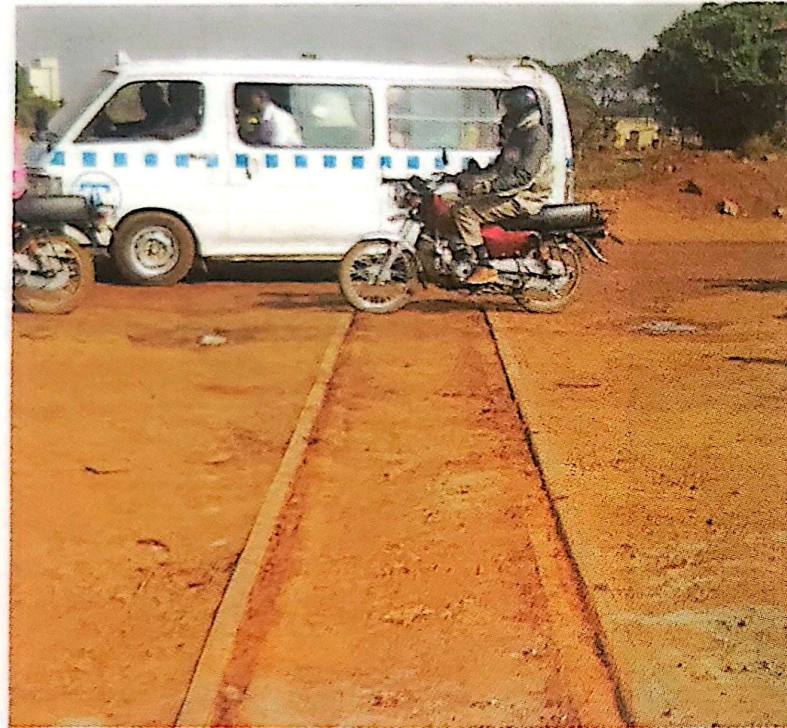
The railway line which has hampered the construction of a drainage system on Engineer Zikusooka Way in Jinja town
