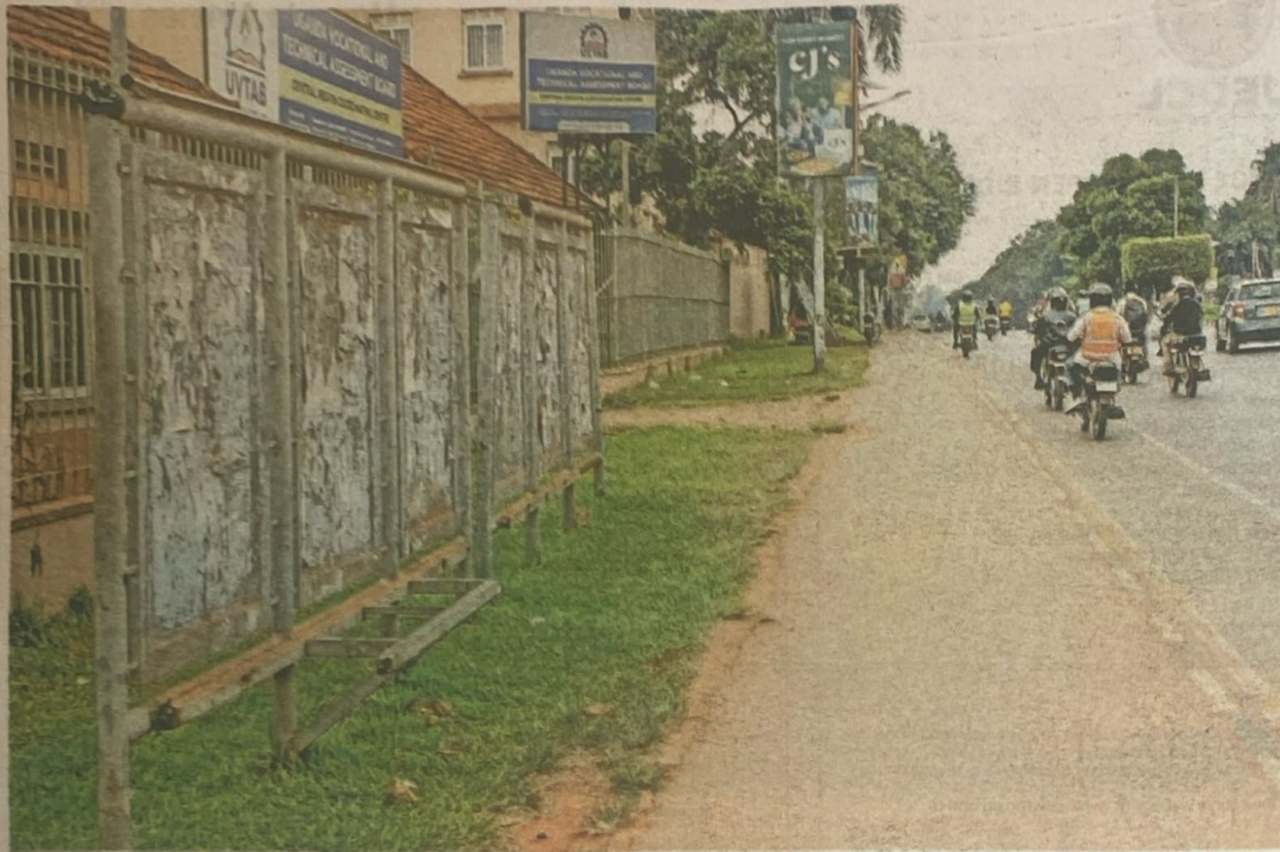
What remains of a once-functioning taxi stage shelter in Kampala. Metal railings have been uprooted, signage stripped, and shelter removed, likely sold as scrap. Commuters now wait in open roadside conditions. PHOTO/GEOFFREY OYET OKWERA
