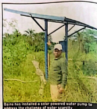
Baine has installed a solar powered water pump to address the challenge of water scarcity
