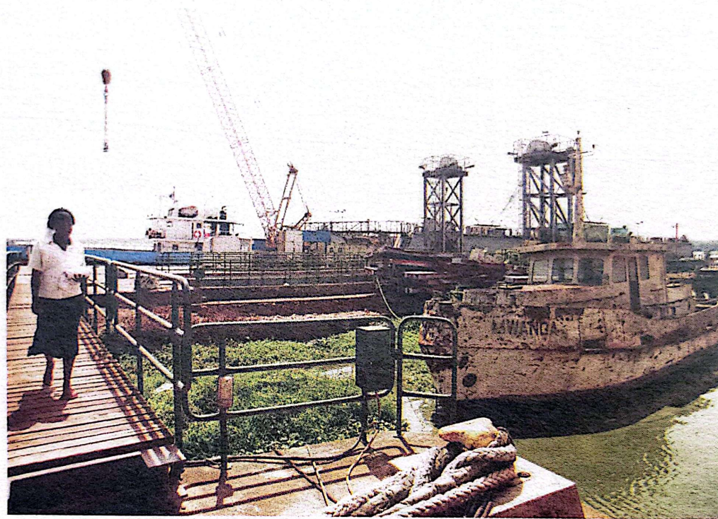
Dilapidated. Port Bell on Lake Victoria was constructed by the colonial government. PHOTO BY RACHEL MABALA
