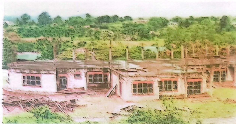
The current state of the stalled Fort Portal City administration block. PHOTO/ ALEX ASHABA
