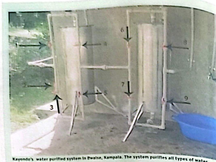
Kayondo's water purified system in Bwaise, Kampala. The system purifies all types of water
