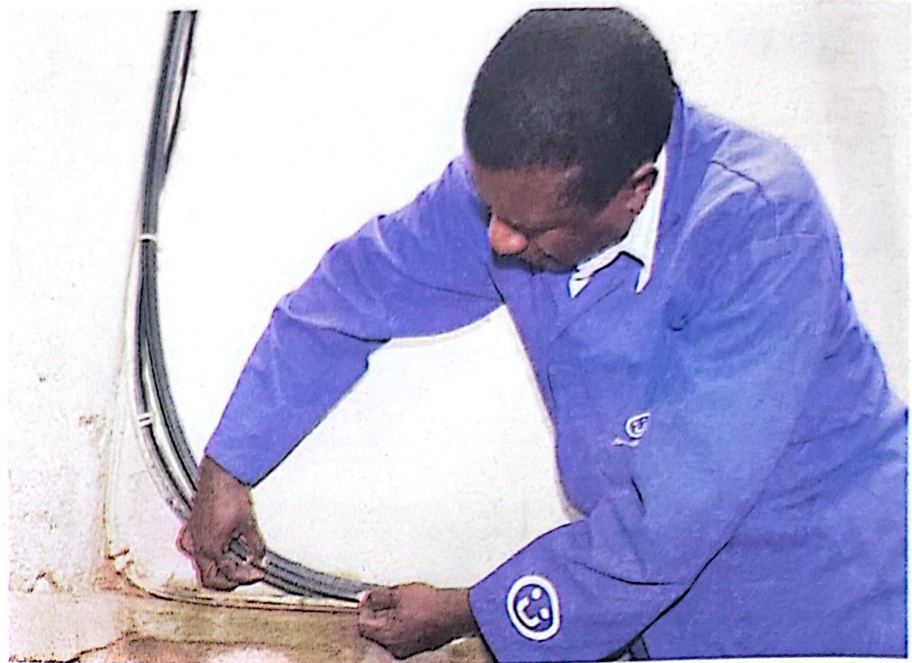
Mr Samuel Wasswa, a Uganda telecom optical fibre technician shows a point where their fibre wires were illegally connected to those of Roke Telkom in Namuwongo, Kampala on Monday. PHOTO BY MICHAEL KAKUMIRIZI
