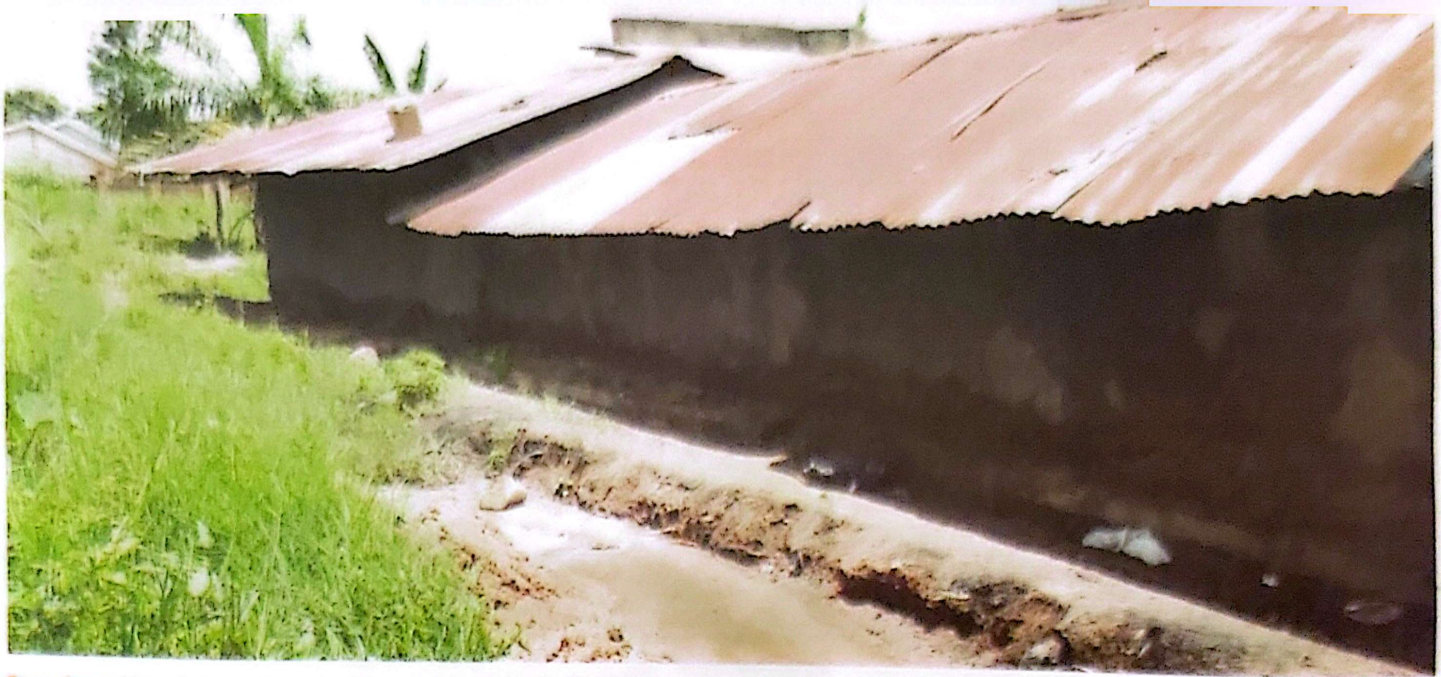
Encroachment. A house that was built in a wetland in Gurua Cell, Arua Municipality. Many people in Arua District are encroaching on wetlands because of rapid urbanisation, which has led to increase of land prices. PHOTO BY CLEMENT ALUMA
