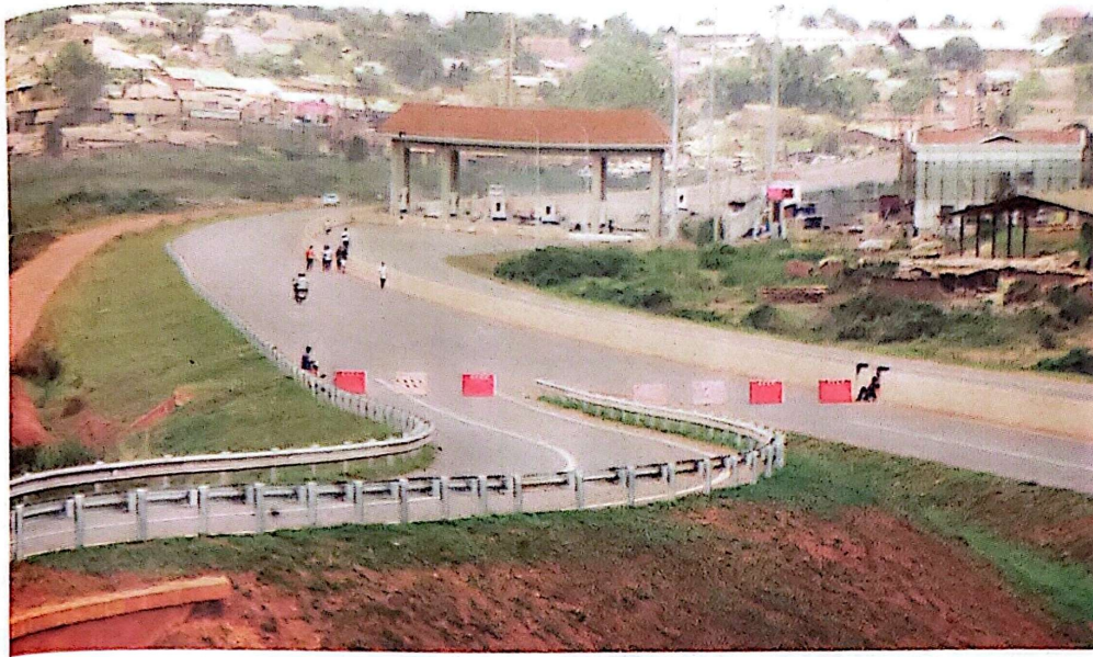
Driving global growth. Entebbe Expressway nearing completion. Infrastructure such as roads drive a country's growth. PHOTO BY RACHEL MABALA
