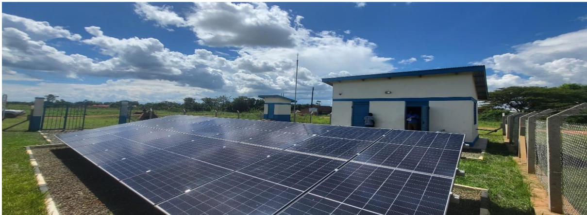
Figure 2 showing the lay of solar panels
