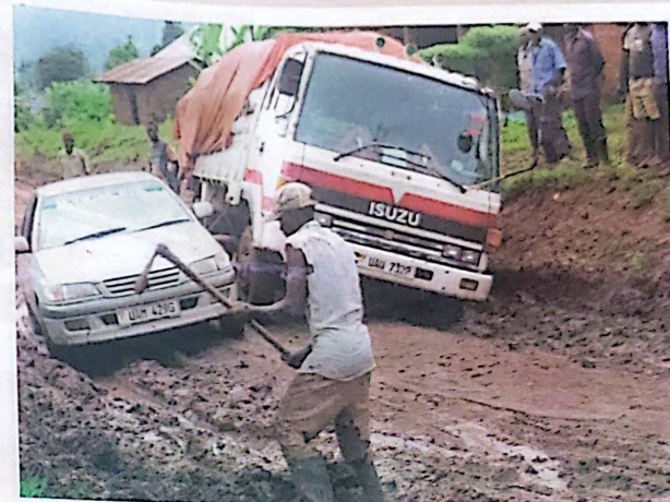
A man attempts to dig vehicles out of the mud along the Namugamba-Budadiri Road to Mt Elgon. PHOTO BY DAVID MAFABI
