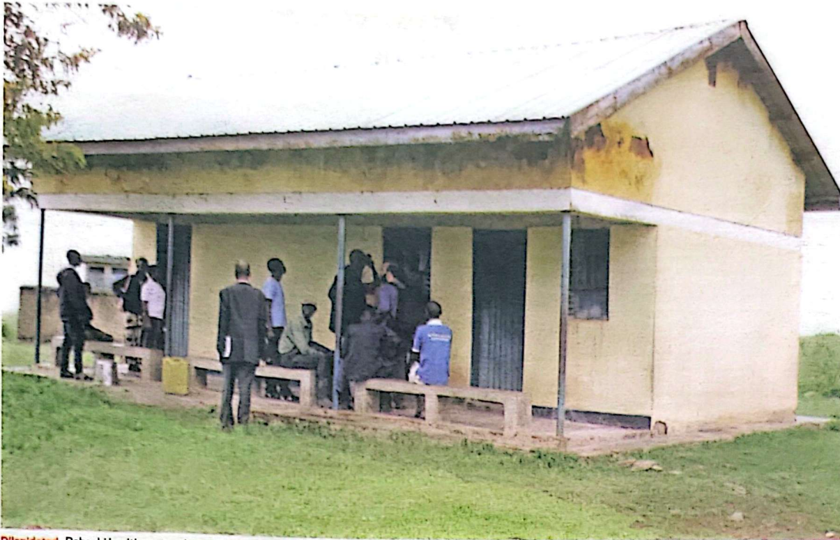
Dilapidated. Rabachi health centre, the only health facility in Rabachi Island, was abandoned because of its poor state. PHOTOS BY RONALD SEEBE
