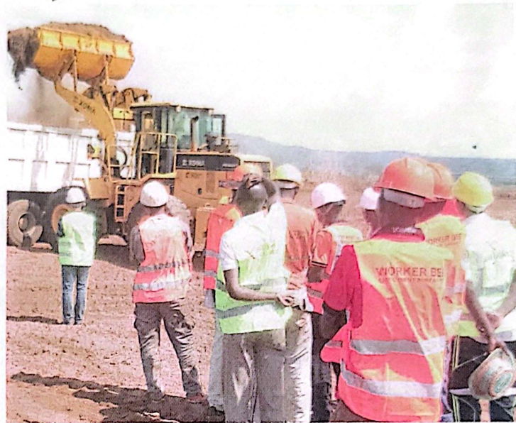
The site where various factories are going to be constructed by Guangzhou Dongsong Energy Group Company Limited, being cleared in Tororo. Photos by Donald Kiirya
