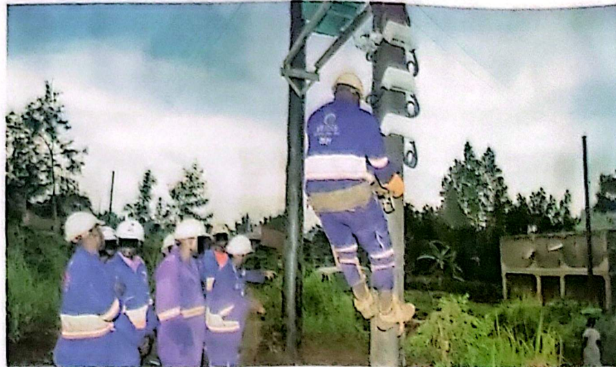
Uganda Electricity Distribution Company Ltd staff go about their duties recently. PHOTO/FILE
