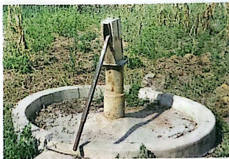
An abandoned borehole in the district
