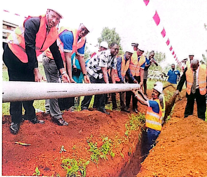
Officials from the water ministry and AfDB laying a pipe. Photo by Agnes Nantambi
