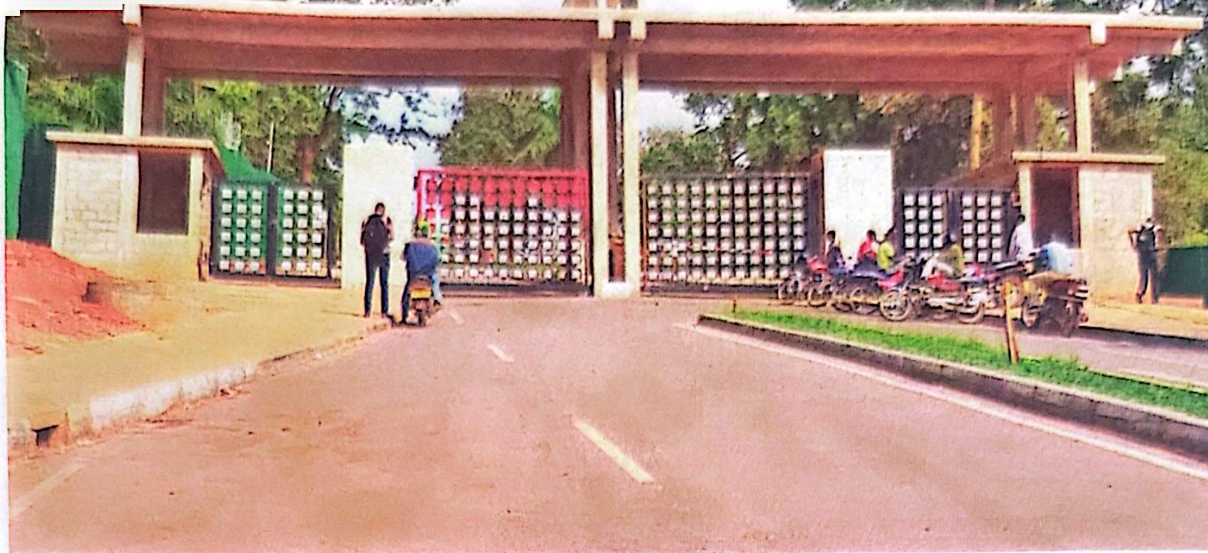
Pending. Makerere University main gate that is still under construction. PHOTO BY MICHAEL KAKUMIRIZI
