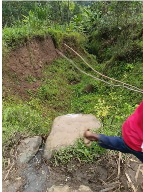
Plate 1: A landslide scarp and erosion channel on a steep hillside, showing exposed soil left by slope failure.
