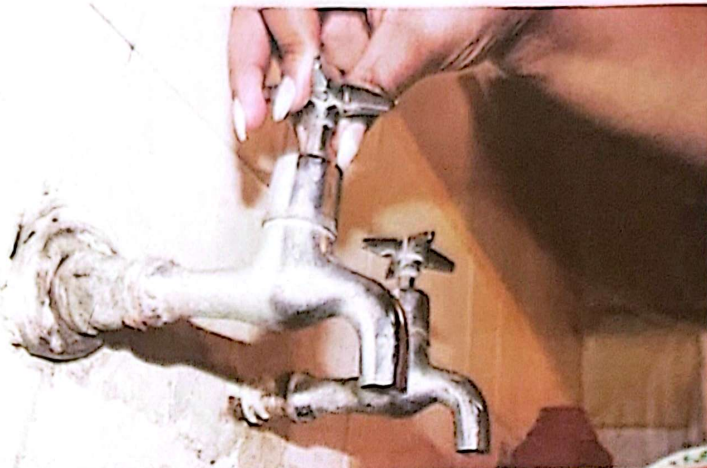
Out. Dry taps at Tenor Estate in Nairobi. AFRICA REVIEW PHOTO
