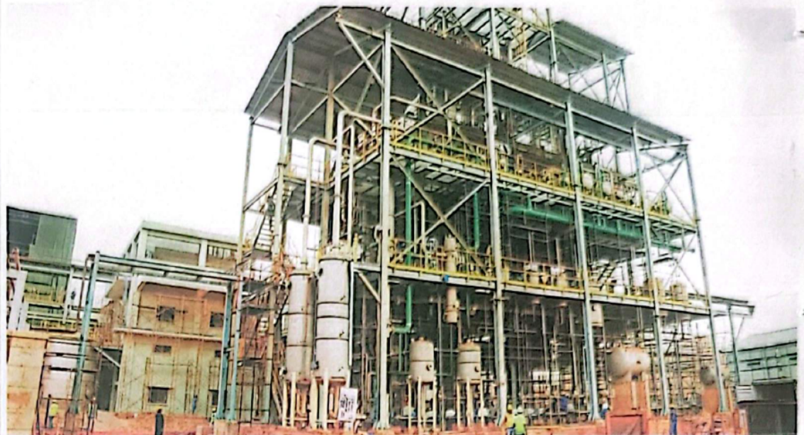
The equipment used to convert bagasse into electricity at Kakira Sugar Ltd factory in Jinja. The electricity generated is not only used within but is also synchronised with the national grid, allowing surplus power to be distributed to surrounding communities and industries. PHOTO/DENIS EDEMA.
