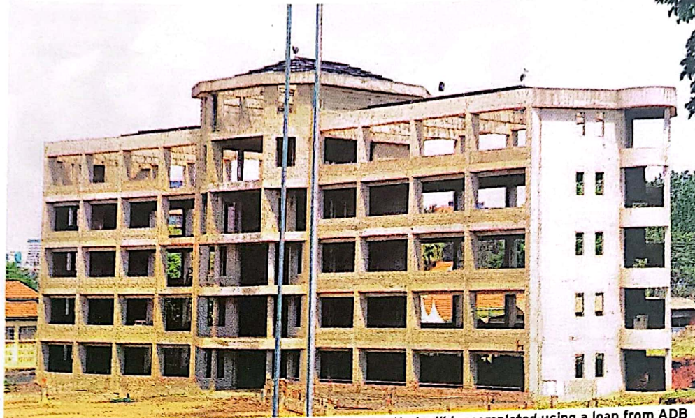
The stalled building at the Uganda Management Institute that will be completed using a loan from ADB
