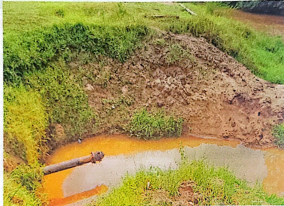
Exposed pipes as a result of the falling water levels. Photo by Abdulkarim Ssengendo
