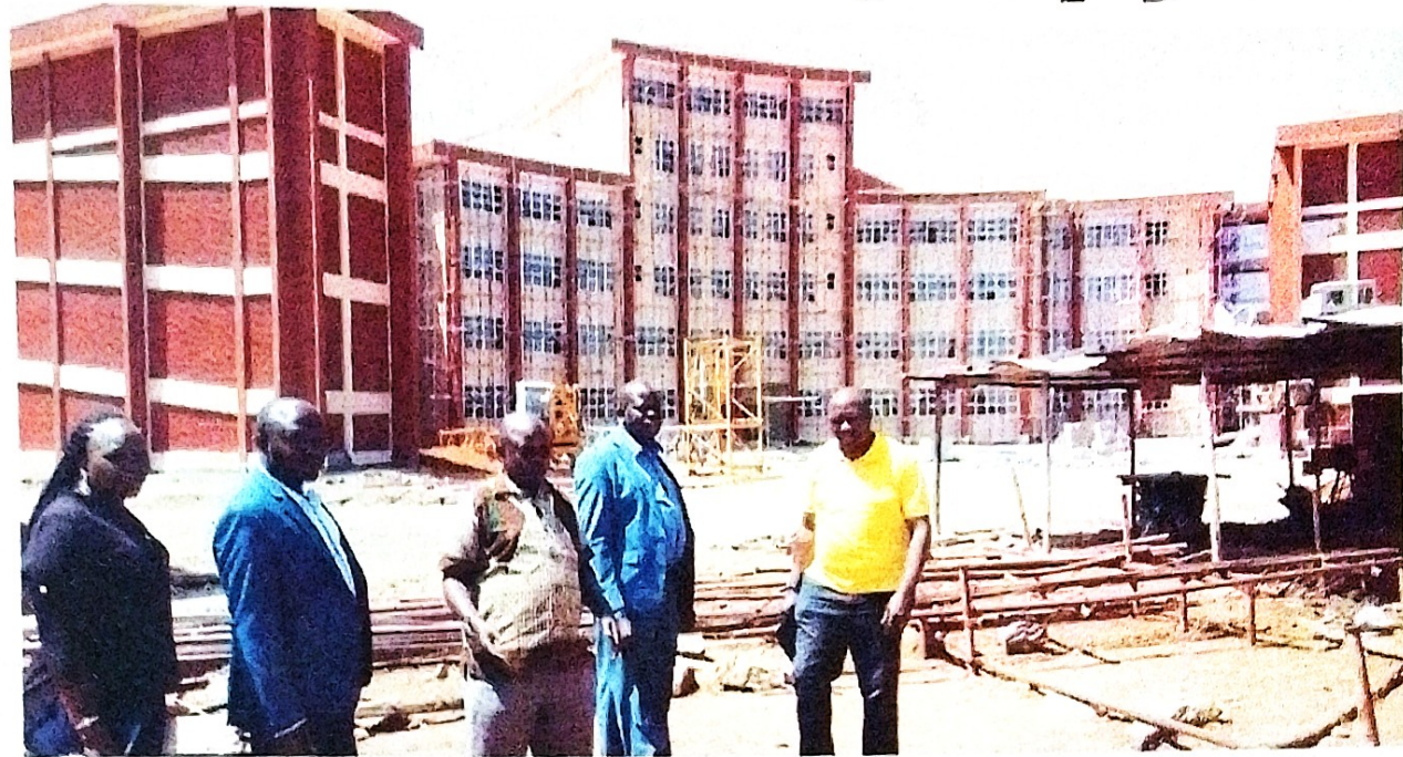
Inspection. Officials inspect ongoing construction works at Soroti University last week. PHOTO BY SIMON EMWAMU
