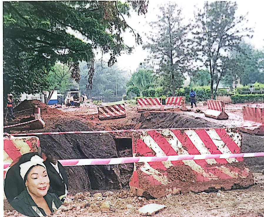
Soqea workers, the National Water and Sewerage Corporation contractors, at Centenary Park where work to install underground sewage pipes was put on hold following a stand-off between Nalongo Estates, the managers of the Centenary Park, National Water and Sewerage Corporation and Kampala Capital City Authority. Inset is Kizito
