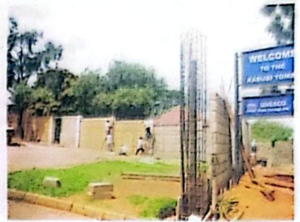
Done. Workers put final touches on the perimeter wall around the tombs. PHOTO BY JOSEPH KIGGUNDU
