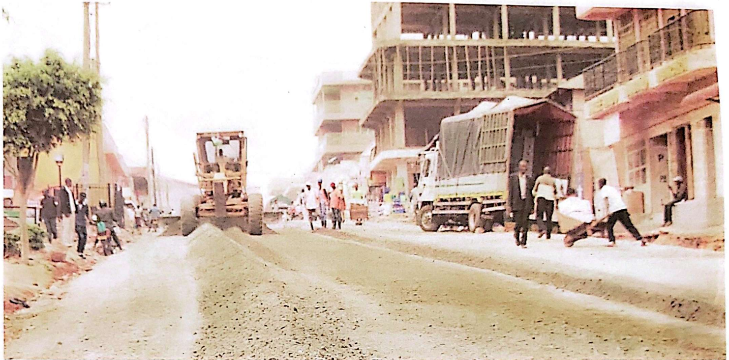
Busy. Engineers lay concrete on Mbaguta Street Road on Tuesday. The project is funded by the World Bank (WB) Uganda Support to Municipalities Infrastructure Development (USMID) Batch II. PHOTO BY FELIX AINEBYOONA
