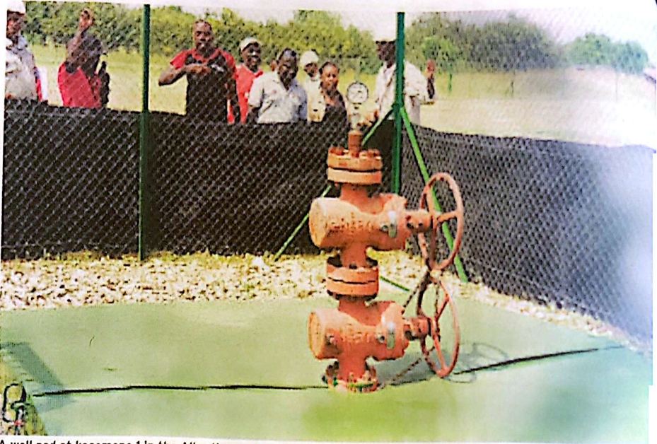
A well pad at kasemene 1 in the Albertine graben, Bunyoro region. Photos by Richard Sanya
