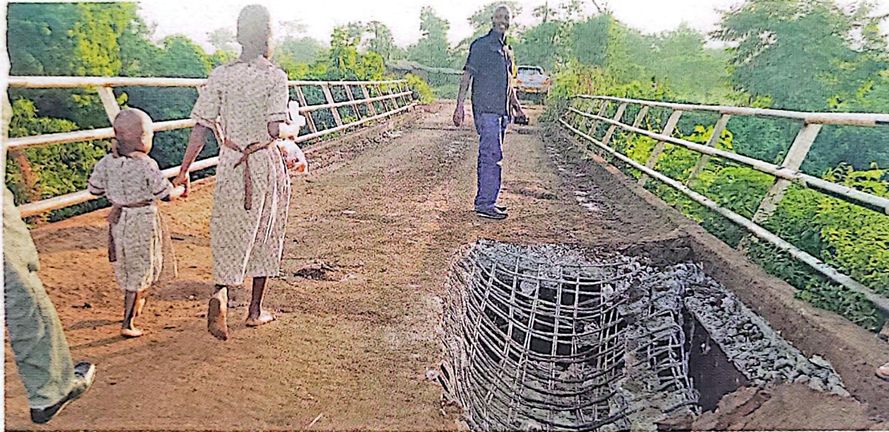
Children walk past the damaged Cheptui bridge along Muyembe-Nakapiripirit highway. Photo by Daniel Edyegu
