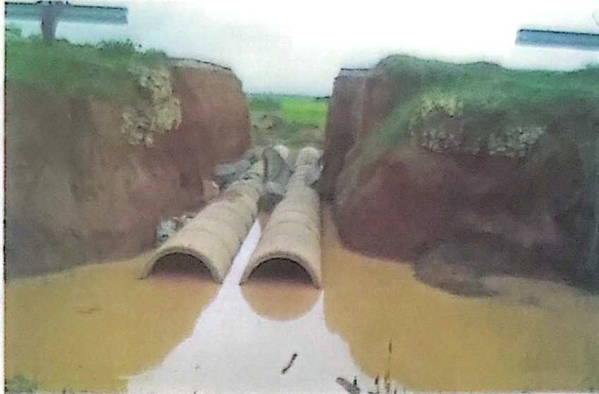
Shoddy work. One of the open water channels that were dug by Dott Services before its contract was terminated. (PHOTO BY FRED WAMBEDE)
