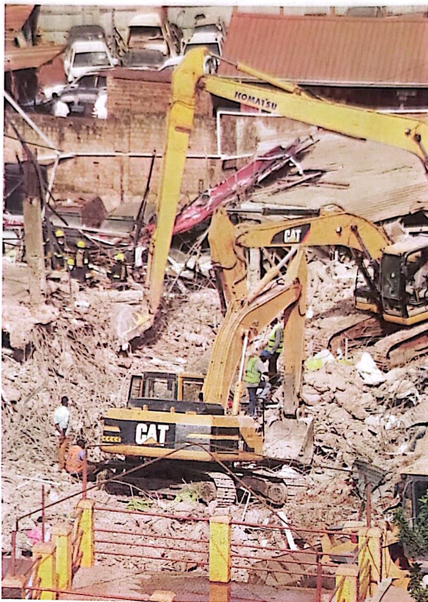
A building that collapsed in Kampala last year due to the use of poor building materials. PHOTO BY ALEX ESAGALA
