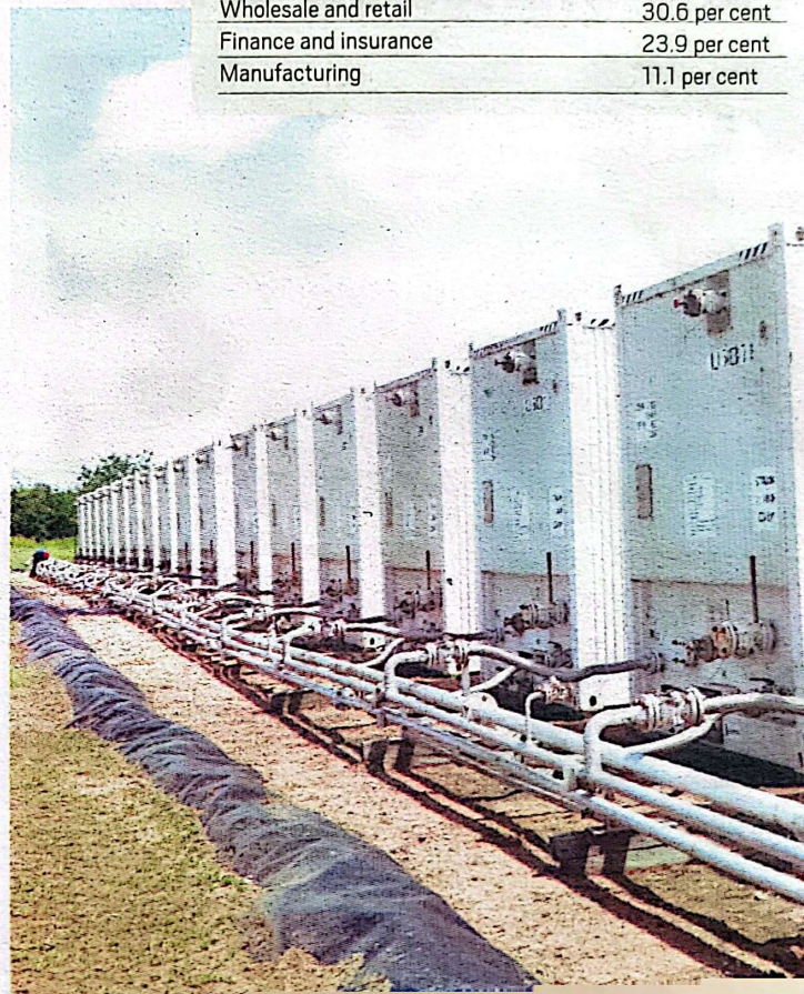
Crude oil tanks at Kingfisher oil well in Hoima District. Such facilities have seen investment in the oil sector surge since 2015. PHOTO BY ERONIE KAMUKAMA
