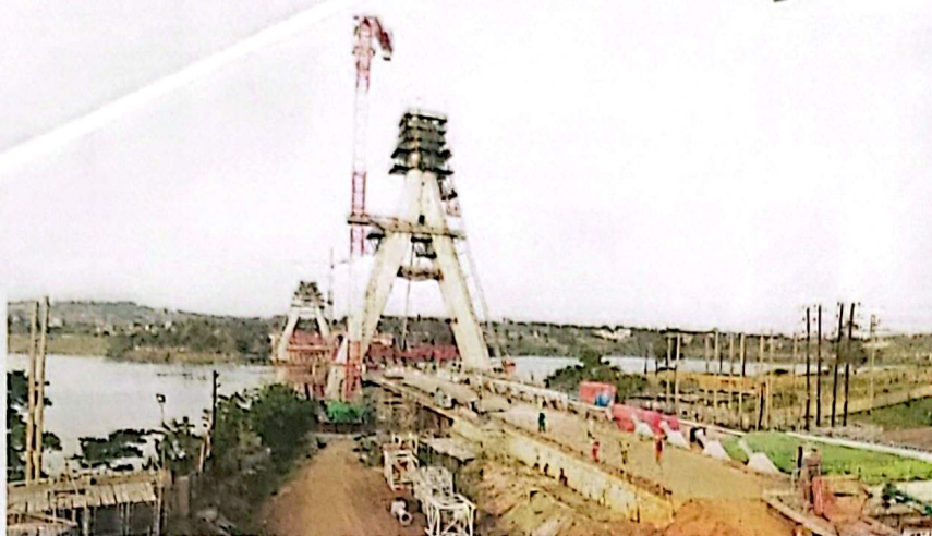
An aerial view of the construction works at the new Nile Bridge from the Njeru side
