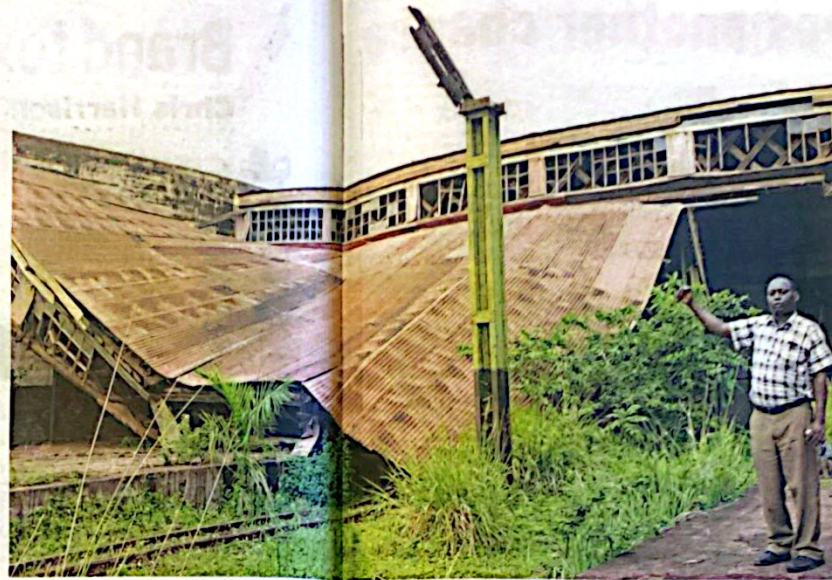
Nicholas Kakeza, an engineer with URC, conducting a tour of a collapsed roof at a train yard in Kampala. Photo by Maria Wamala
