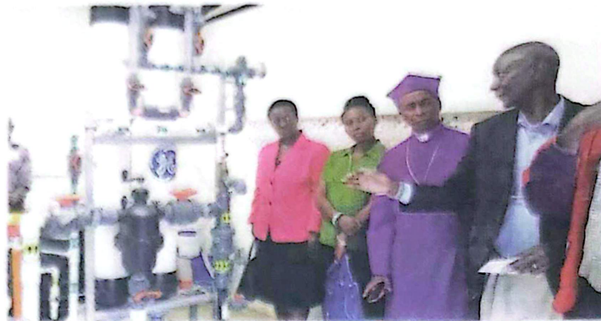
Bishop Zoreka and other officials inspecting the newly commissioned water filtration system. Photo by Agnes Nantambi
