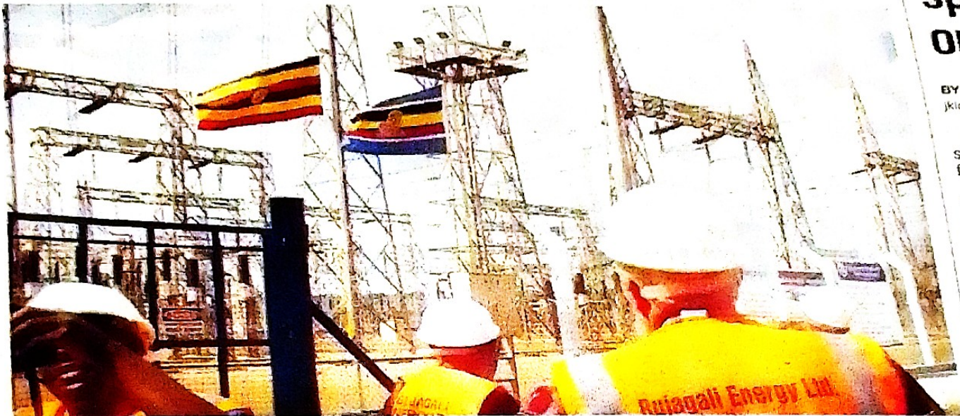
Electricity centre. A section of Bujagali Hydropower Station. PHOTO BY JOSEPH KIGGUNDU
