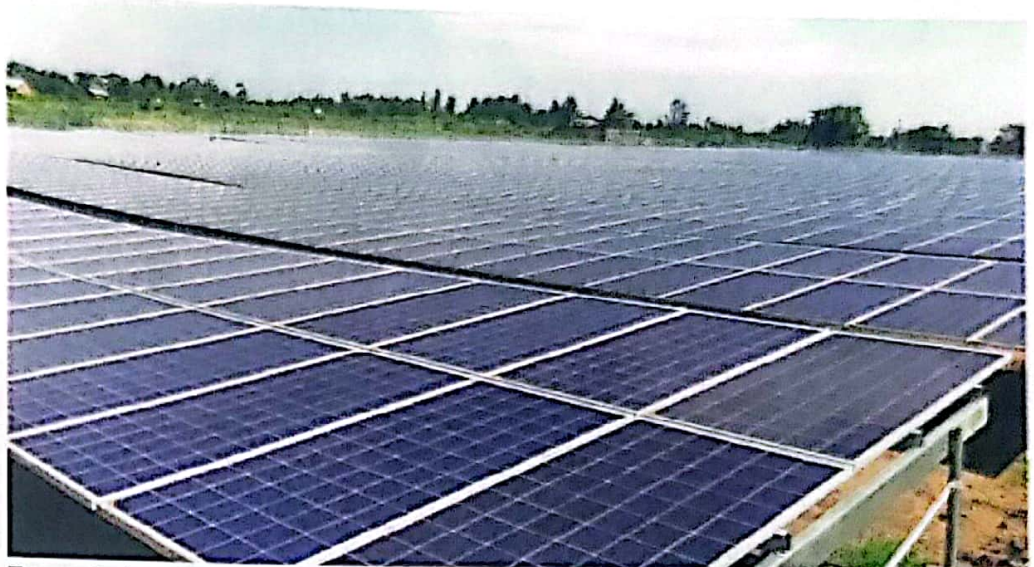
Tororo Solar North power plant is undergoing performance tests by UETCL and Umeme
