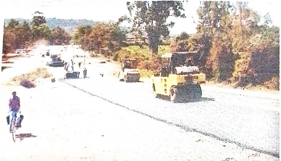
Projects. Road works underway. Infrastructure projects such as roads usually take up the biggest chunk of money borrowed by government. FILE PHOTO
