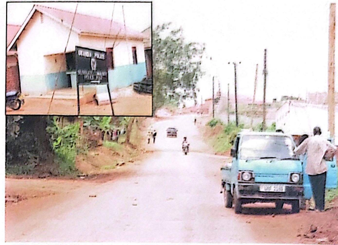
Buwaate Road, which is being constructed by the community. Inset is the Police station the community fundraised for and built. Photo by Ramadhan Abbey
