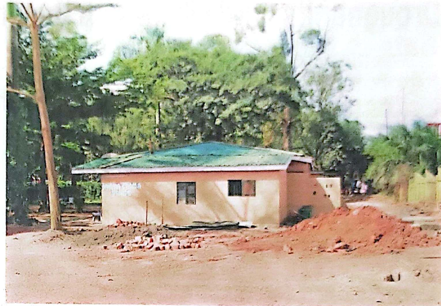
The Nyama Choma Place that has been constructed on top of the National Water and Sewerage Corporation sewer line in Centenary Park. Photo by Ramadhan Abbey
