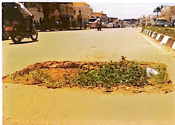
Shoddy. A section of Republic Street, one of the Mbale municipal roads that have been under construction since 2014. PHOTO BY LEONARD MUKOOLU
