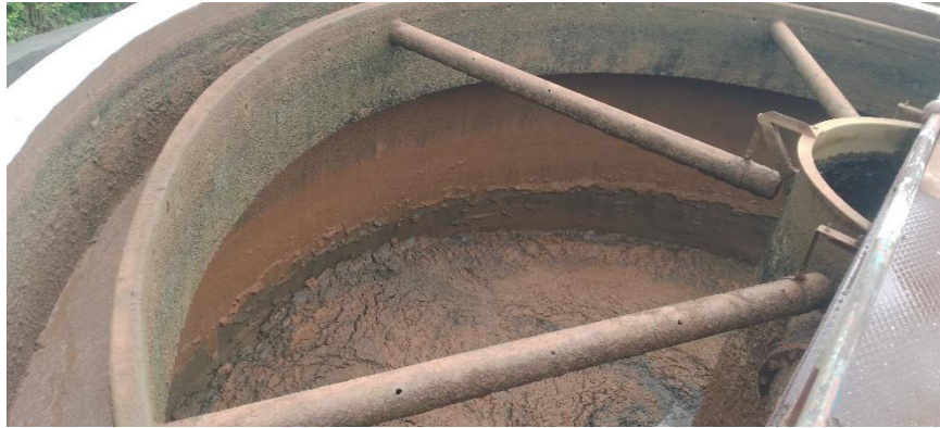
Figure 2.2: Showing sludge in a clarifier
