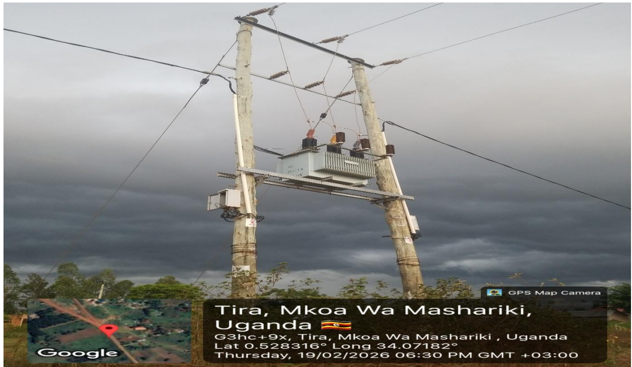
Figure 5-1 50 kVA Ajuket Road TX
