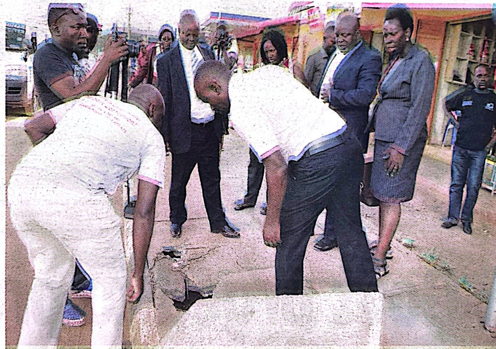
A team from the Inspectorate of Government and the Public Procurement and Disposal of Public Assets in looking at defects on the new roads in Mbarara. Photo by Abdulkarim Ssengendo
