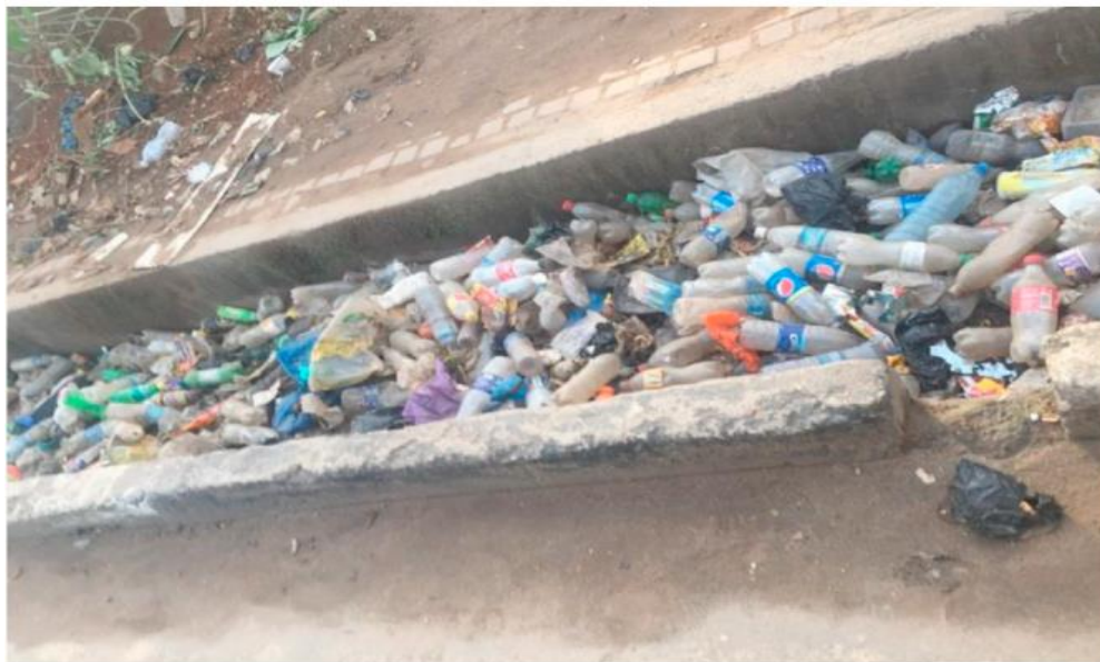
Figure 1.1: Plastic Waste Causing Blockage in Drainage Systems.
