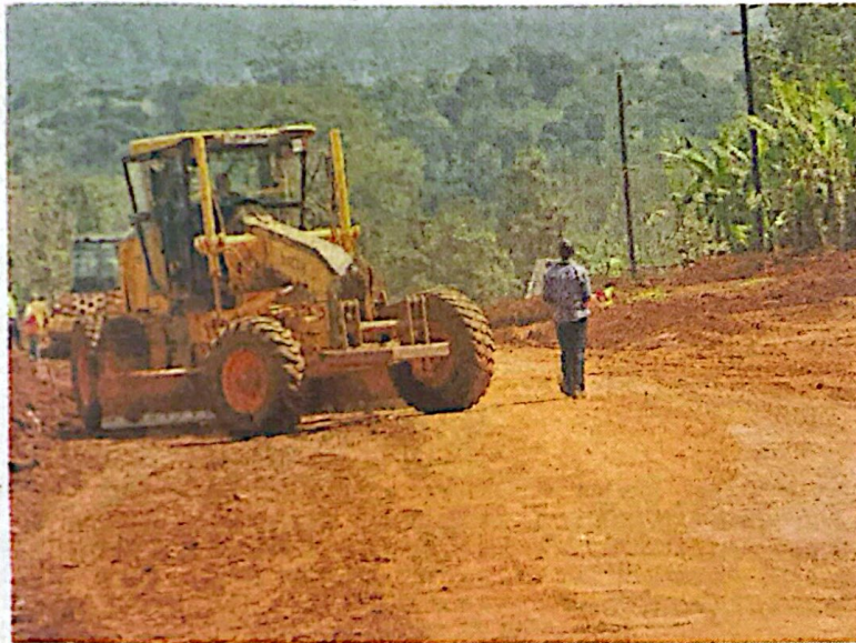
Works on Mukono-Katosi road were halted because of the procurement contract saga between Eutaw Construction Company and Uganda National Roads Authority
