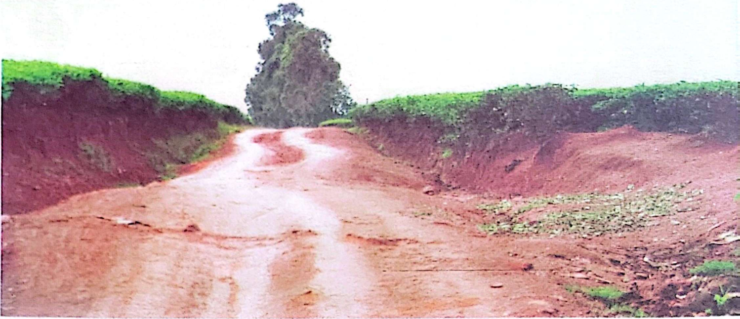
It is important to check if the land you are buying has an access road because you might be left at the mercy of your neighbour. PHOTO BY DAVID S. MUKOOZA
