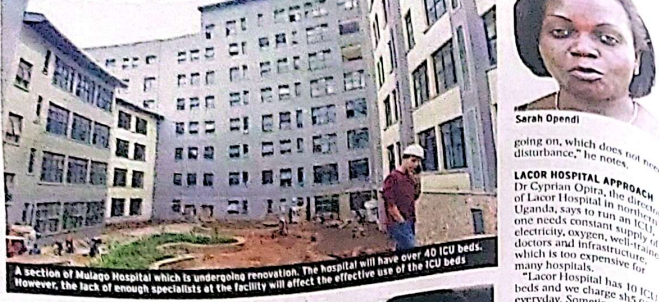
A section of Mulago Hospital which is undergoing renovation. The hospital will have over 40 ICU beds. However, the lack of enough specialists at the facility will affect the effective use of the ICU beds.
