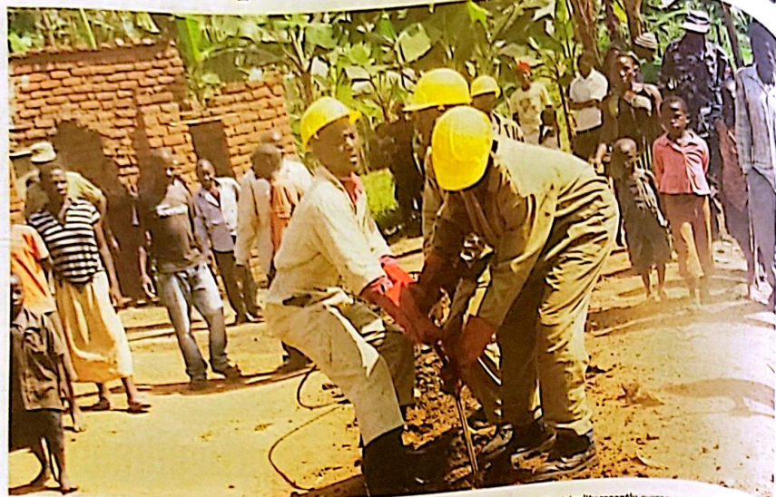
Power loss. Umeme officials uproot power cables used to illegally connect power to people's houses in Doko cell, Mbale Municipality recently. PHOTO BY DAVID MAFAYI
