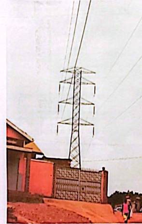
High voltage. Umeme installs transformers in many trading centres so that electricity from high-voltage lines such as these is altered to levels that households can use. PHOTO BY ABRAHAM LUBWA
