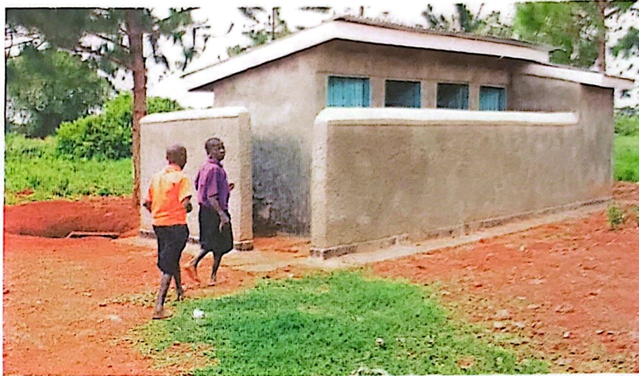
The poorly constructed pit latrine at Kasozi Primary School has attracted criticism from the residents. Photo by Geoffrey Namukoye
