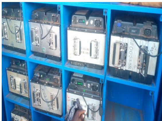
Figure 9: Batteries on charge
