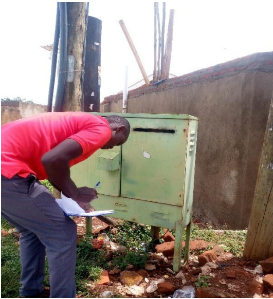
Figure 5: Transformer meter reading and recording
